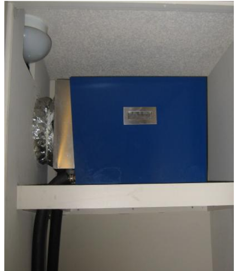
Geyser mounted in a closet
